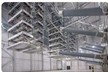
A rare look inside one of the Western Link valve halls where the AC (alternating current) electricity that is used on the main network is transformed into DC (direct current) electricity to allow it to be transferred efficiently through the long cables.
