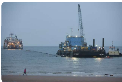
Cables being pulled ashore at Ardrneil Bay in Scotland through ducts under the beach
